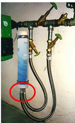
The activator installed underneath the water tap with connections facing downwards .
